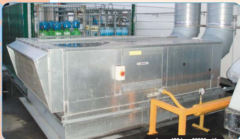
make-up 408 kw - 30000 m 3 /h
